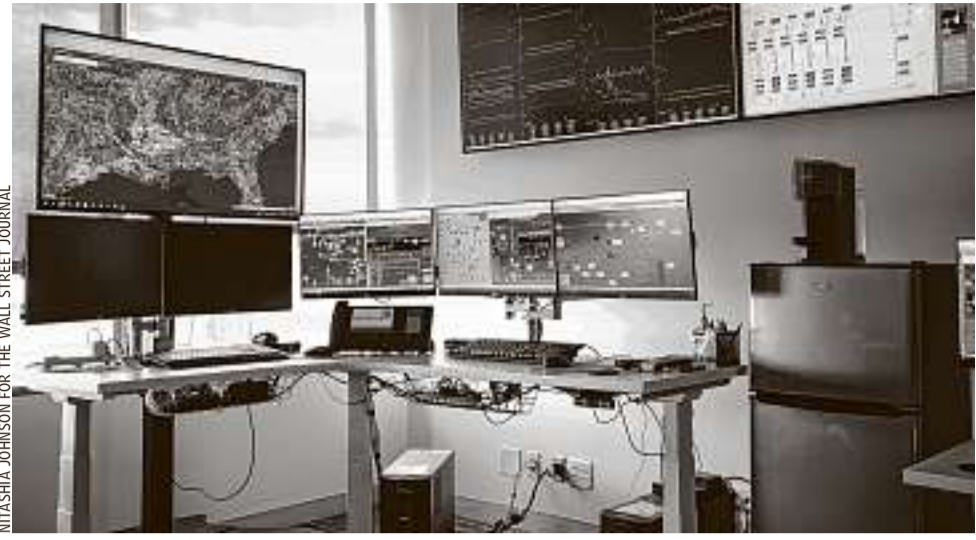
Denbury's pipeline-control center in Plano, Texas. The company has miles of pipelines in several states.
